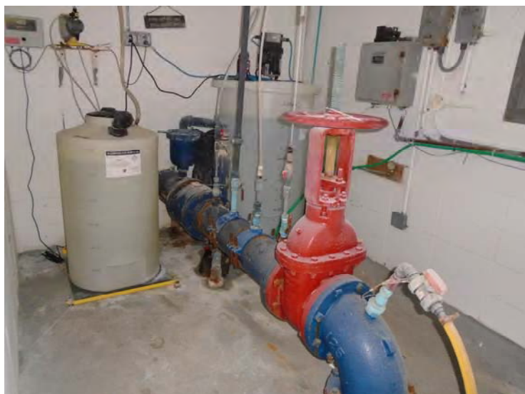
37. The piping is located in the control building; the coating is in fair condition.
