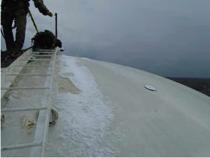
23. The exterior roof coating is in poor condition.
