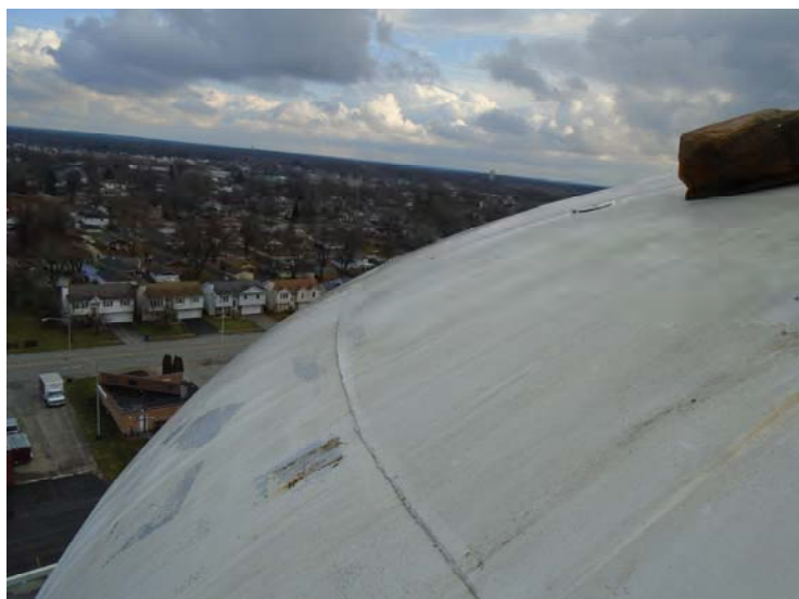
22. The exterior roof coating is in poor condition.
