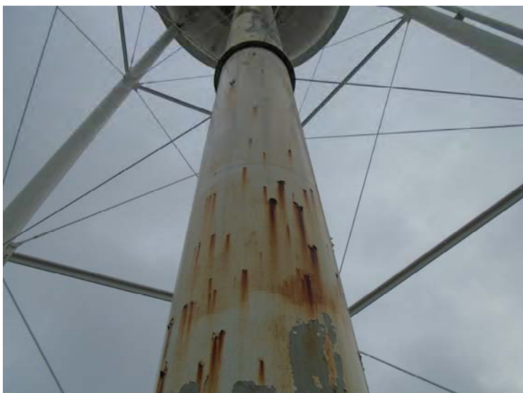
13. The exterior riser coating is in poor condition.
