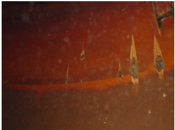
30. Areas below the water level are covered with heavy mineral staining.
