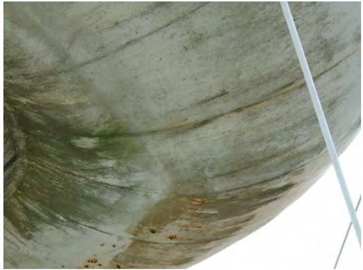
15. The exterior bowl coating is in poor condition.
