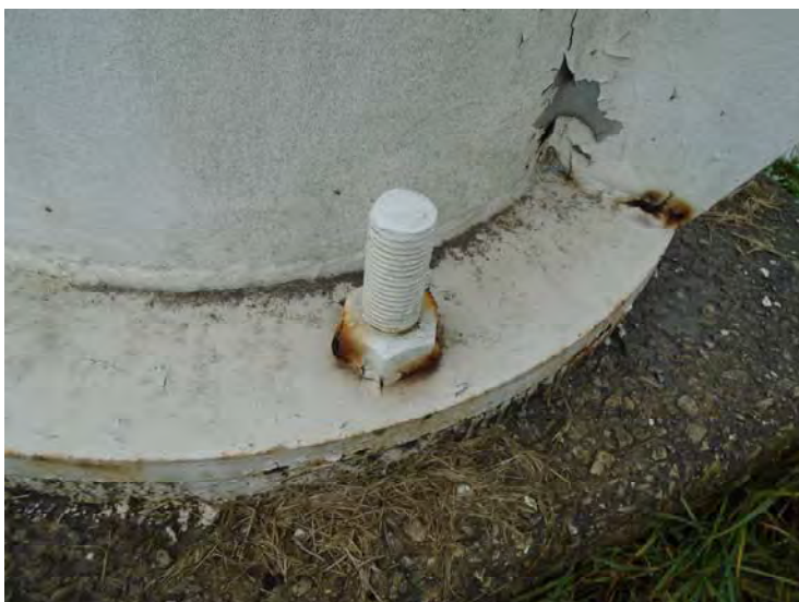
4. The exterior leg anchor bolt coating is in poor condition.
