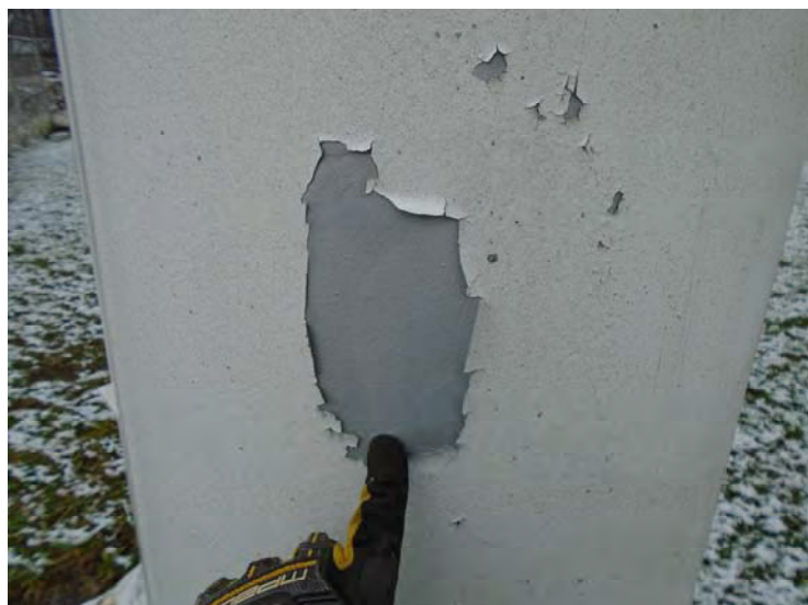
7. The exterior leg coating is in poor condition.
