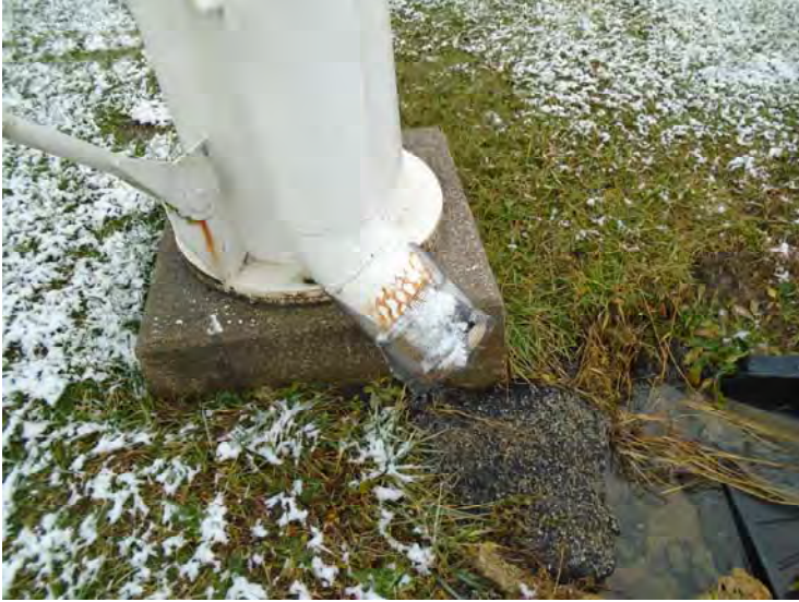
5. The exterior overflow pipe coating is in poor condition.
