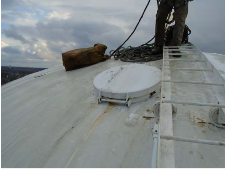
26. The wet interior roof hatch coating is in poor condition.
