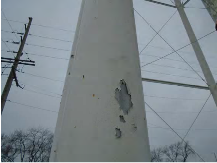
8. Extensive topcoat delamination was found on the legs.
