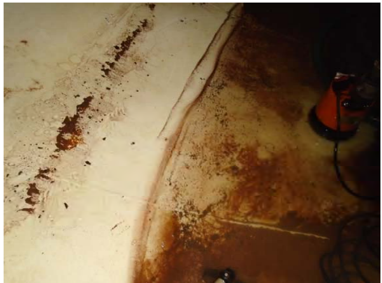
33. The wet interior bowl coating is in fair condition.
