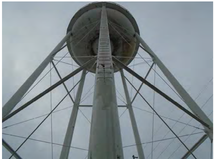
9. The exterior leg ladder coating is in poor condition.
