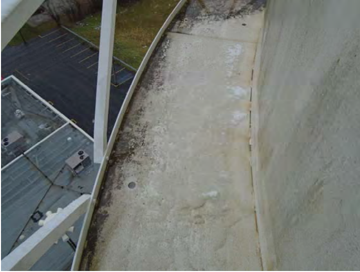
17. The exterior balcony coating is in poor condition.
