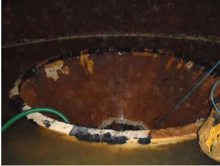
35. The wet interior riser transition cone coating is in poor condition.
