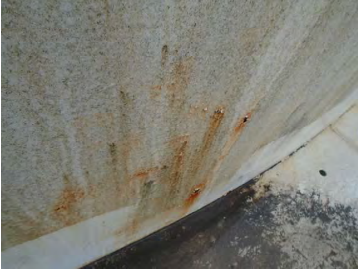
20. Extensive rust bleedthrough was found on the sidewall.
